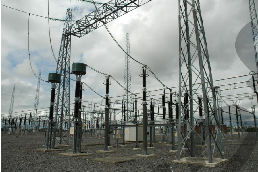
Figure 3.1: Typical AIS Equipment
